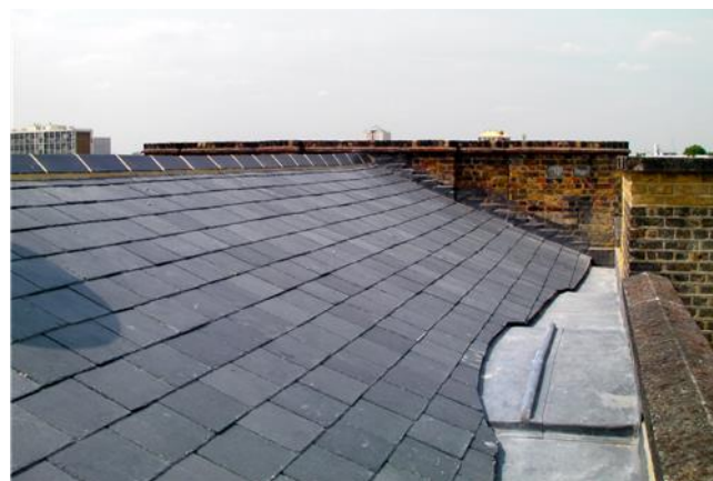
Roofs were re-slatted (original slates were re-used on the front slope), lead gutters, parapet walls and copings were restored; roof trusses were strapped
